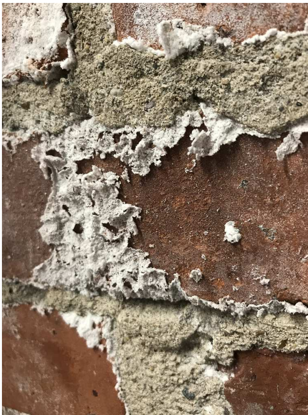
Figure 5.1: Heavy efflorescence on brickwork. These bricks were originally covered with efflorescence, most of which has flaked off. (This photo was taken in my chemistry lab where these bricks form part of the chimney for the building.)
